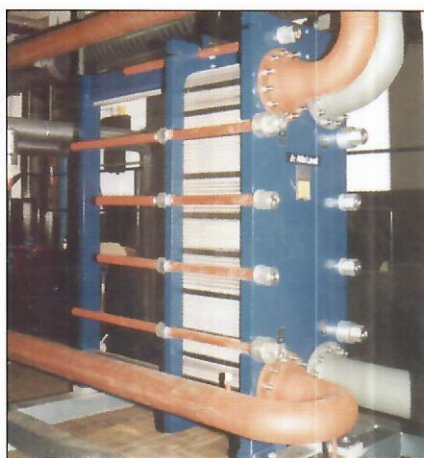
Fig. 2 SWPHE as an evaporator in a brewery installation.
